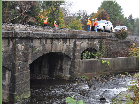
Members of the Project Team conducted an inspection of the NHHS Rail Line on October 19, 2011 and stopped to examine the stone arch bridge over the Mattabasset River in Berlin.
